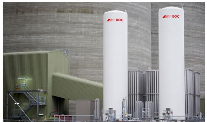
BOC Biomass Fire Suppression system
